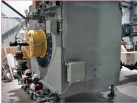
New Indeck Burner
